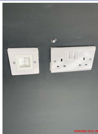
White plated double plug socket. In good and clean condition.
