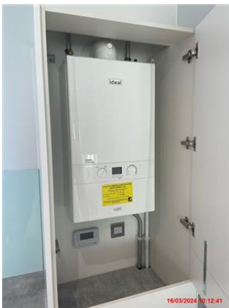
Ideal boiler inside of cupboard to corner of kitchen. Boiler in good condition.
