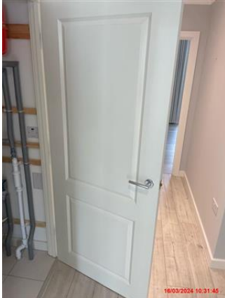
White wooden door. Chrome handle - intact. In good condition. Door sturdy.
