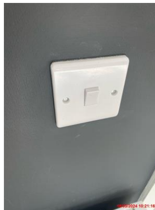
White plated single light switch. In good and clean condition.
