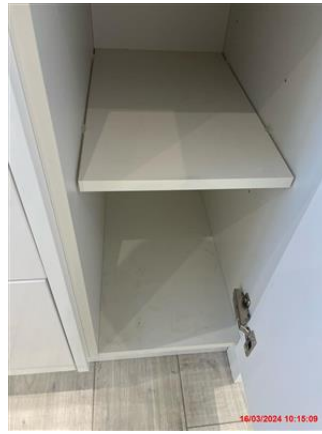
Stains to bottom shelf of cupboard.
