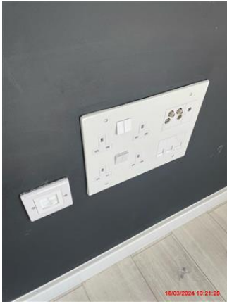
White plastic switch/aerial connection sockets. In good condition.
