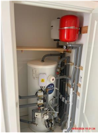
Water tank cupboard. Water tank in good condition.
