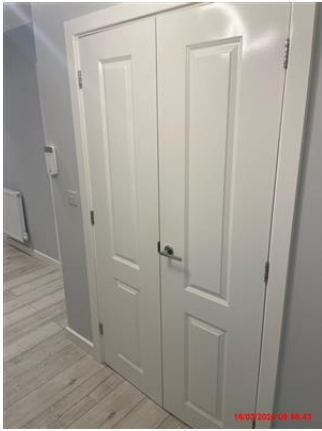
White wooden doors. Chrome handle - intact.
