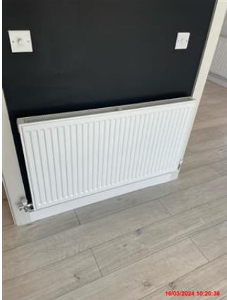
White double panel radiator. In good and clean condition. Temperature control caps intact.
