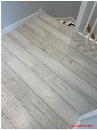
Grey laminated flooring. Floorboards intact. In clean condition. In overall good condition.
