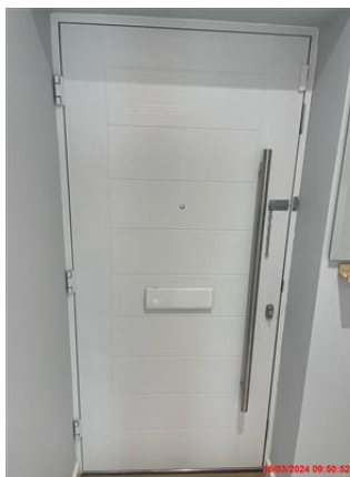
Reverse side of door white. Chrome handle to match exterior. Chrome chain lock - faulty Chrome deadlock - intact and functional.
