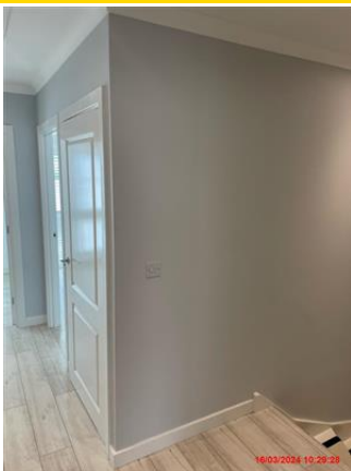
Light grey painted walls. Walls in good condition. Paintwork in good condition
