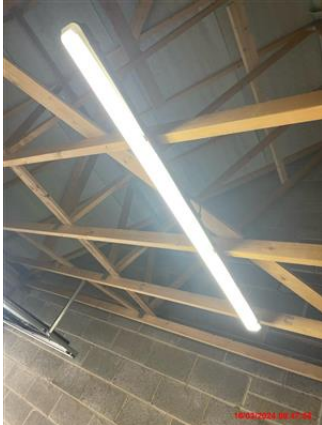
Florescent tube lighting. In working order.
