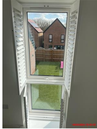
White UPVC windows. Double glazed. White handle – intact. Windows secure. In good and clean condition.
