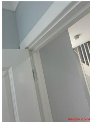
White painted door frames. Frames in good and clean condition. Paintwork in good condition.
