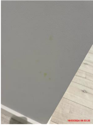
Small sized stains to corner of wall.
