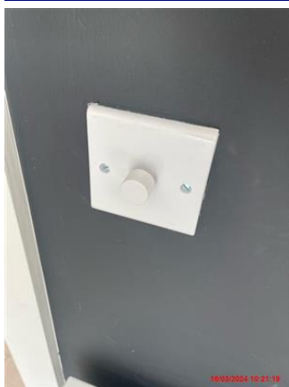
white plastic dimmer switch. In good condition.
