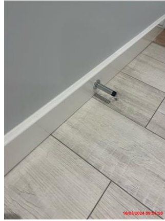
Slight dust to top of skirting. Chrome door stop with black tip - intact.
