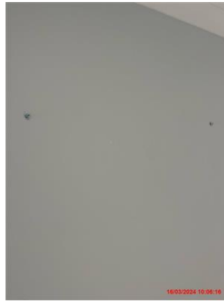
X2 nails in wall.
