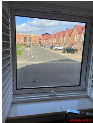
White UPVC windows. Double glazed. White handle - intact. Windows secure. In good and clean condition.
