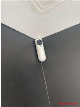
White cased video camera to top corner of wall. Not in use.
