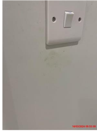
Faint mark to paintwork below light switch.
