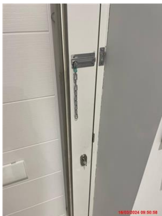
Chain lock faulty as noted.
