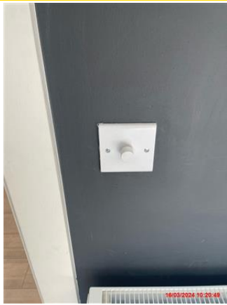
white plastic dimmer switch. In good condition.
